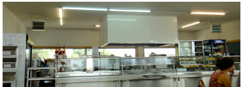
Figure 37 Lighting of Higher School Education cafeteria in Setúbal.
